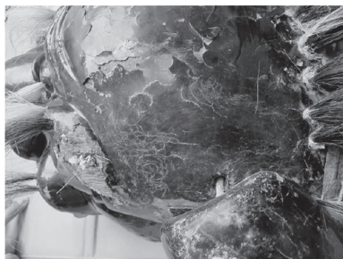
図9 塗膜剥落、剥離、汚れ
